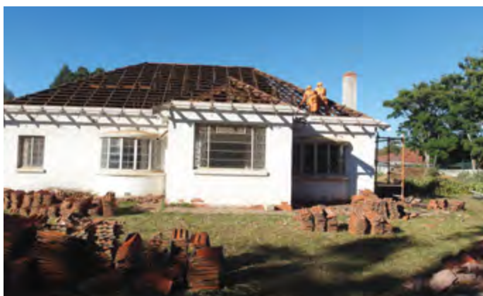
May: Demolition of old structure to make way for the new building
